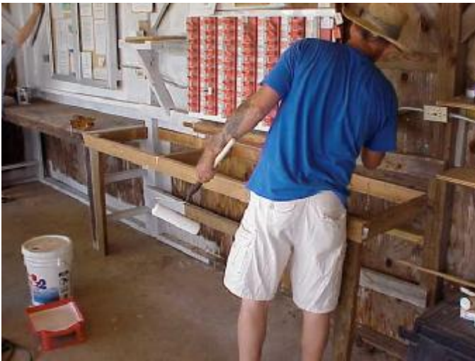
Beginning of new charging table (James)
